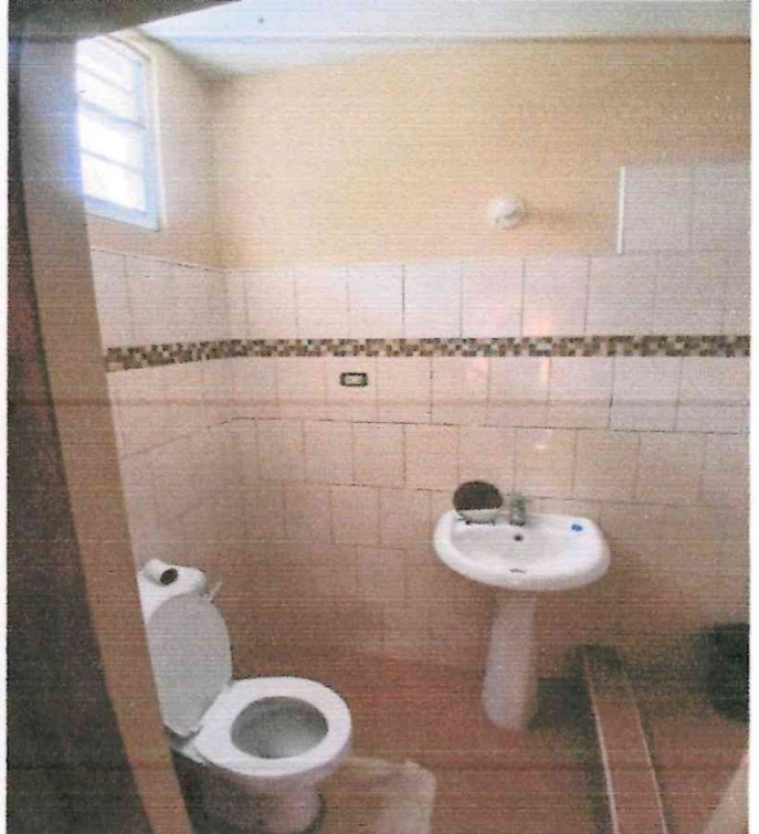
TOILET AND BATH/FACE BASIN
